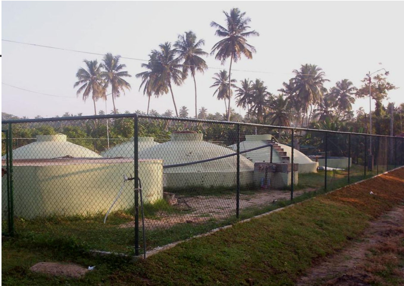
Waste water treatment plant - Negombo
