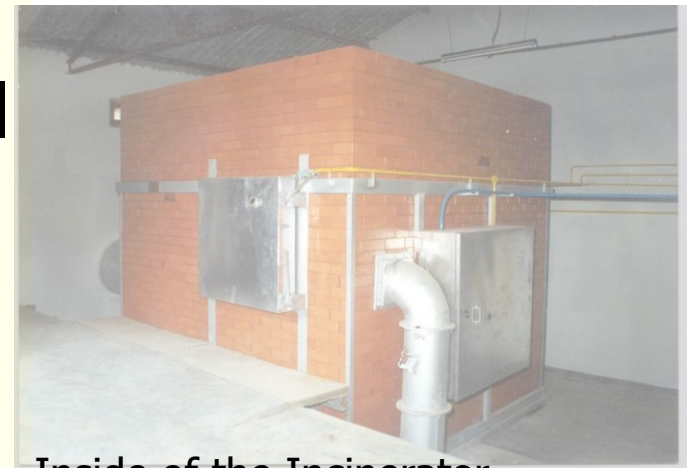
Inside of the Incinerator
