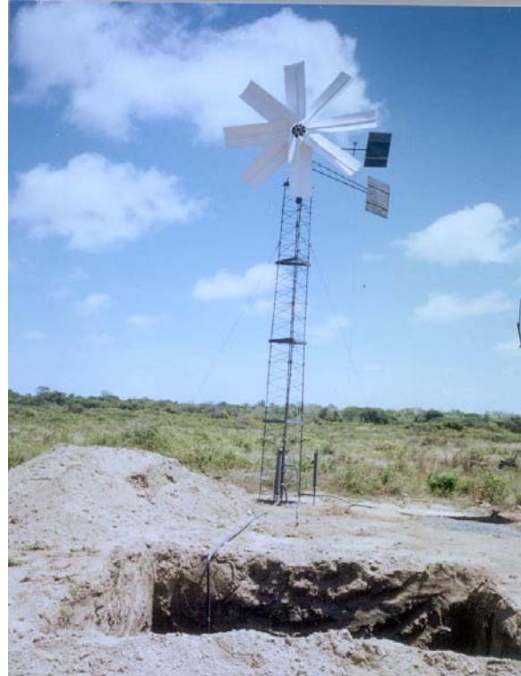
Figure .2: water pumping wind pump, installed in the North Central part (Higurakgoda) of Sri Lanka
