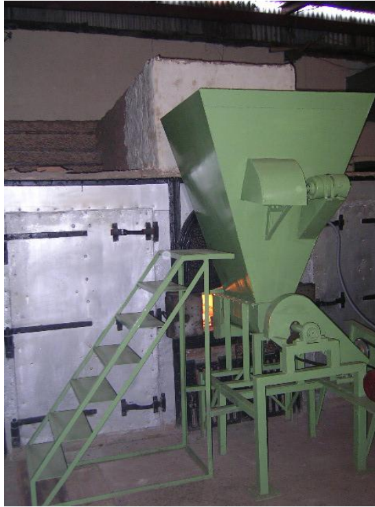
Fig.6. Screw Coveyor Couple to the Existing Furnace
